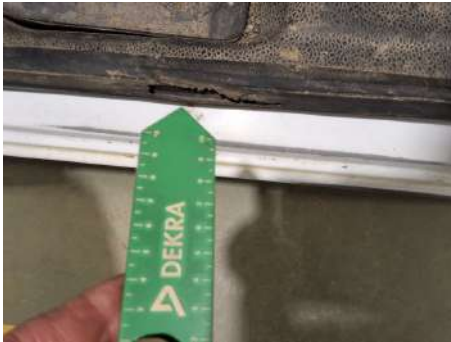
Door entry seal / Front Left / Tear
