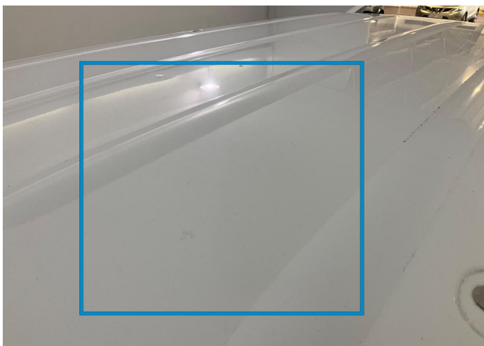
5. Roof Bodywork / Dent / Hail Area -
